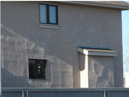
Stucco will crack uncontrollably. These cracks will allow water to get in behind the stucco.
