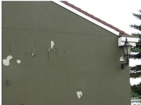
The acrylic stucco failed due to a faulty wall detail, no such failures with rainscreen.
