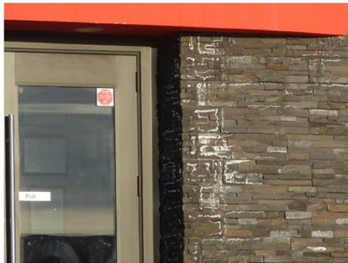
This manufactured stone developed efflorescence. Removal is not possible.
