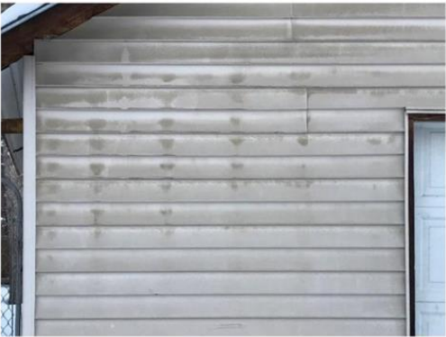
Vinyl siding will attract dirt from the constant expansion and shrinkage. (Static electricity)
