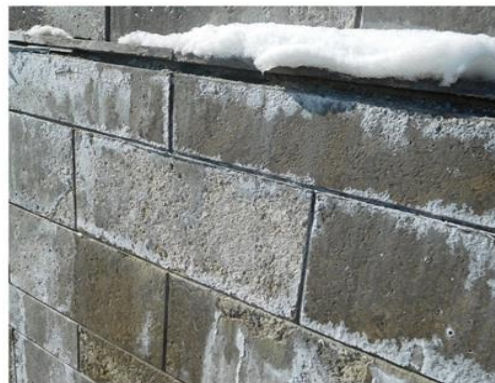
Real limestone panels were mortared onto this wall without drainage. It lasted only 5 years.
