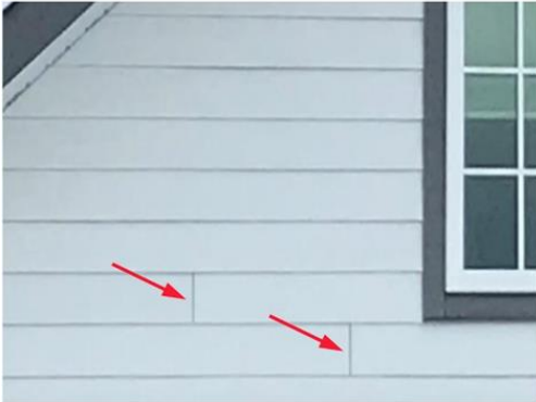
Hardy board panels are often joint together without sealing these joints.
