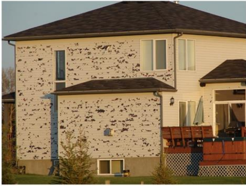
The vinyl siding exterior on this home was destroyed in a hailstorm.
