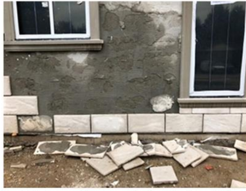
On this home the manufactured stone fell off before the installation was even completed.
