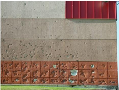
This acrylic stucco was applied over dense insulation and subject to severe vandalism.
