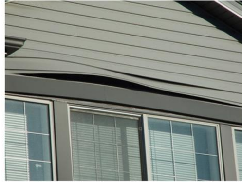
Expansion of the vinyl siding can cause buckling and even popping out.
