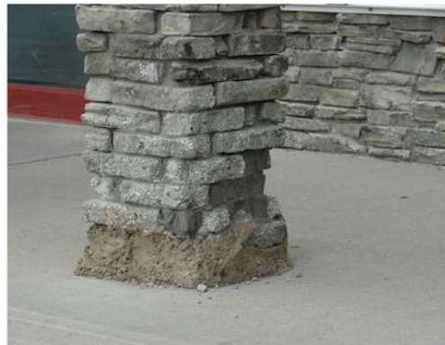
The lightweight aggregate in manufactured stone absorbs water and causes it to fail.
