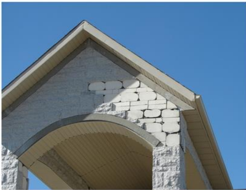
On this home Granite stone panels fell off again, resulting in a dangerous situation.
