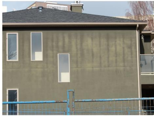
Acrylic stucco was used on this wall which resulted in some unsightly fading.
