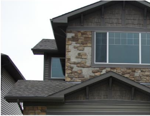
The manufactured stone fell off. Permanent adhesion cannot be guaranteed.
